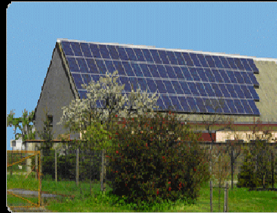
Rooftop integrated PV plant
